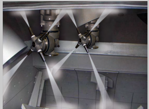
A80R heads installed in a twin-shaft mixer
